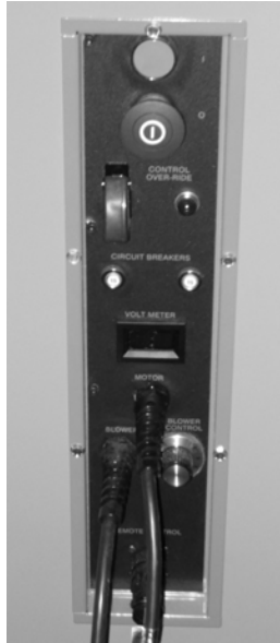
Figure 6 (Blast electrical panel shown)
