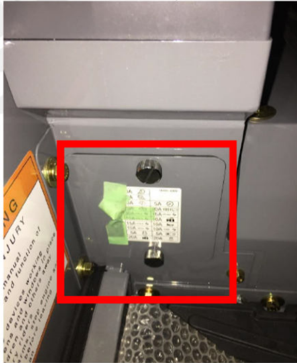
TL8 Uninstalled Fuse Example
