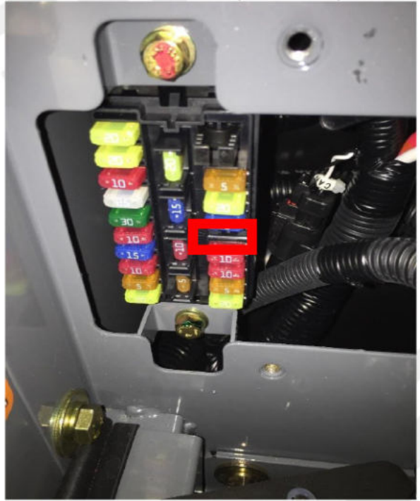
TL8 Uninstalled Fuse Example Cover Open
