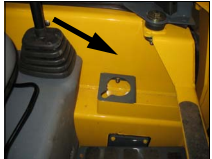
Figure 1 – Fire Extinguisher Location
